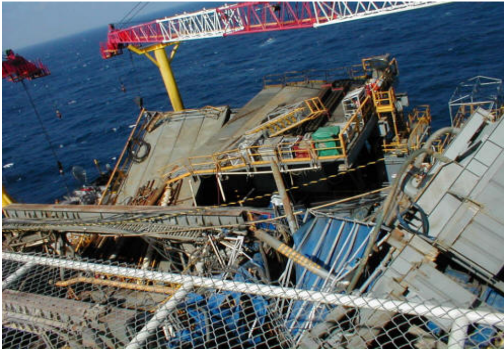
Seven platforms in the Gulf of Mexico destroyed by Hurricane Ivan in 2004
